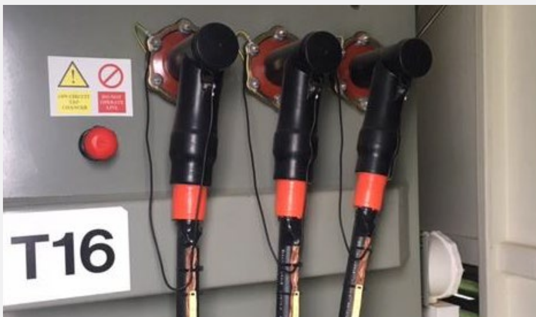
Figure 15 – Isolation boots – Faulty installation can cause safety hazards
